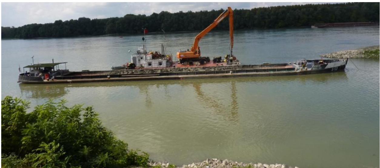
Figures 5-8: Dredging on the Danube with a bucket dredger working with a float
